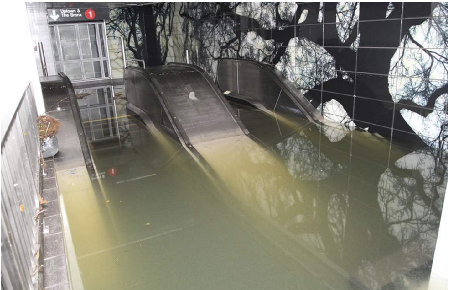
Fig 13.3 Flooding Damage to a Subway Station in Lower Manhattan
