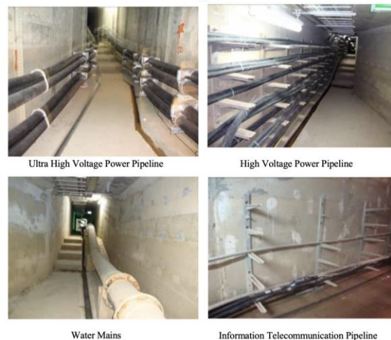
Figure 5. The Utilidor of the High-Speed Rail in Taoyuan City
