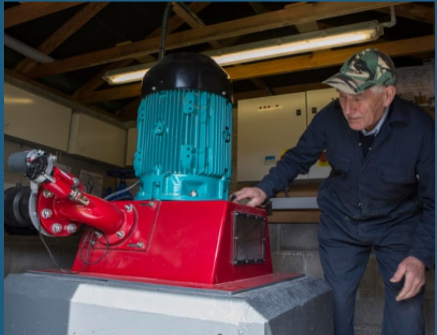
Figure 8: Howell Williams checks on his small diversion hydropower system. Source: The Guardian 39
