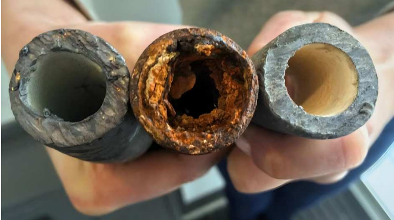
Figure 5. Examples (from left to right) of a lead pipe, a corroded steel pipe, and a lead pipe treated with protective orthophosphate ( U.S. EPA Region 5 )
