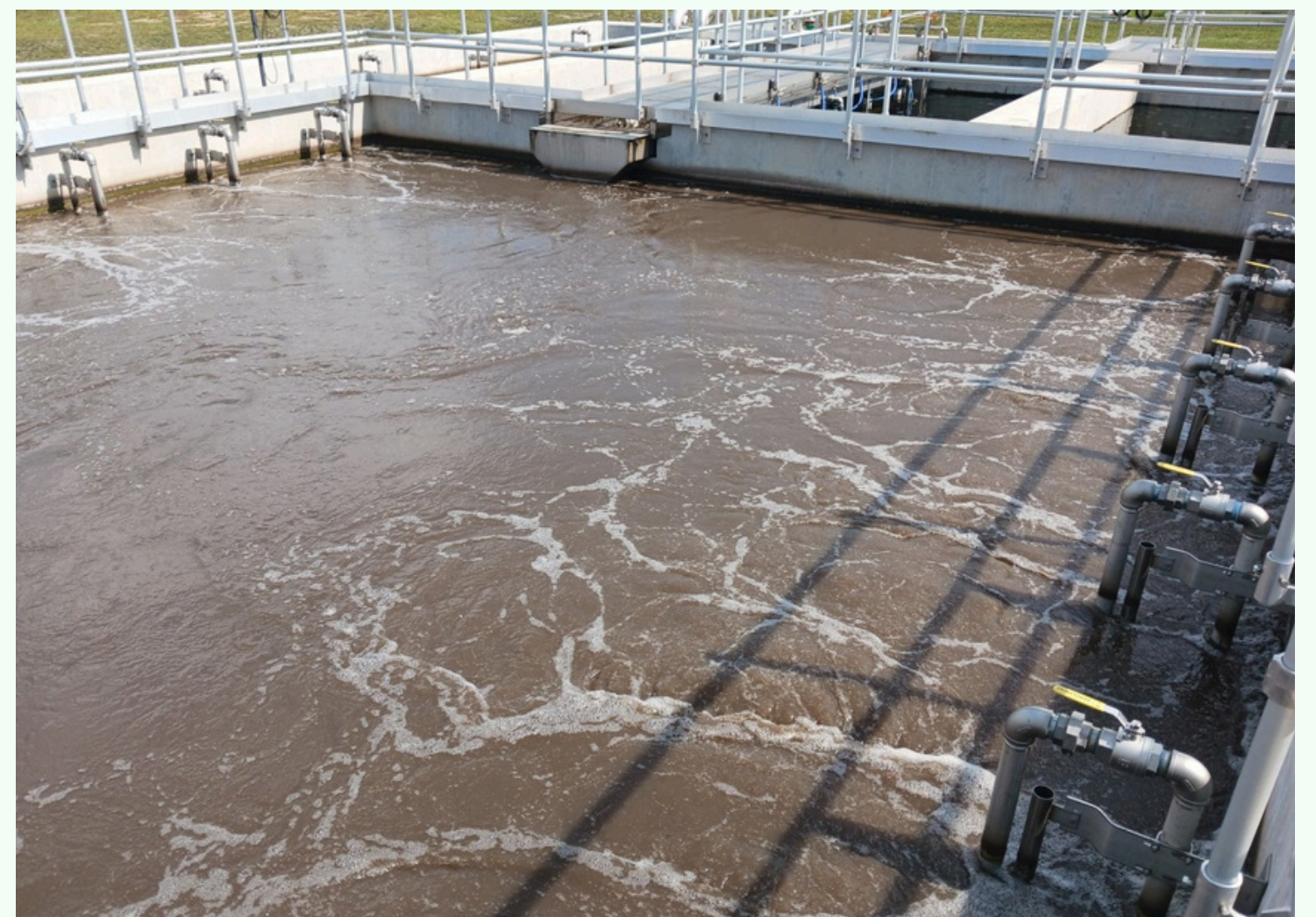
Figure 15: Activated-sludge Aeration Tank Treating Textile Effluent
