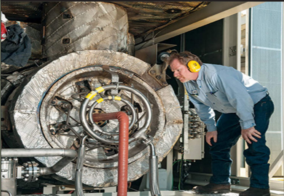
Figure 6. A turbine generator at a East Bay Municipal Utility District wastewater treatment plant, driven by biogas to generate
