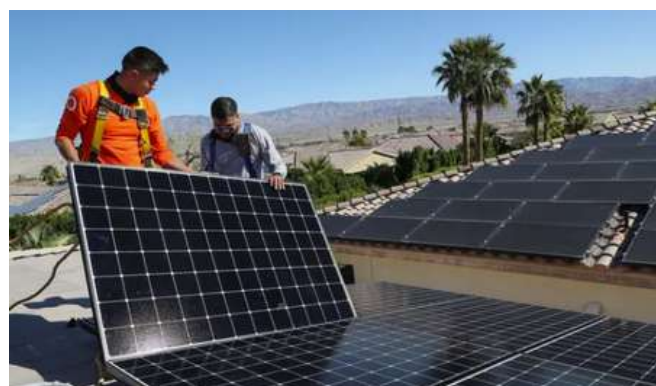
Renova Energy Solar Project via Jay Calderon
