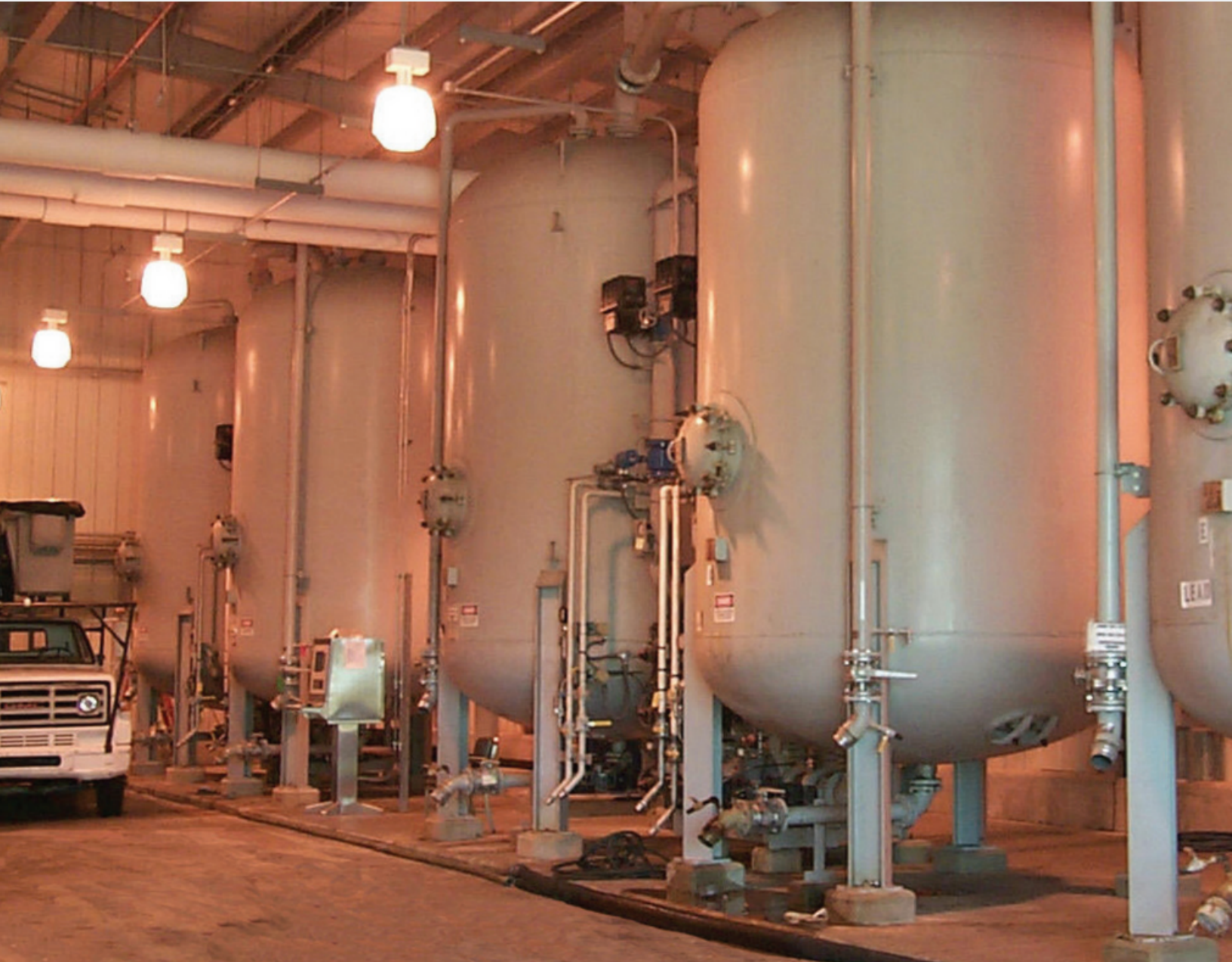
Tanks of granular activated carbon Source: U.S. Environmental Protection Agency
