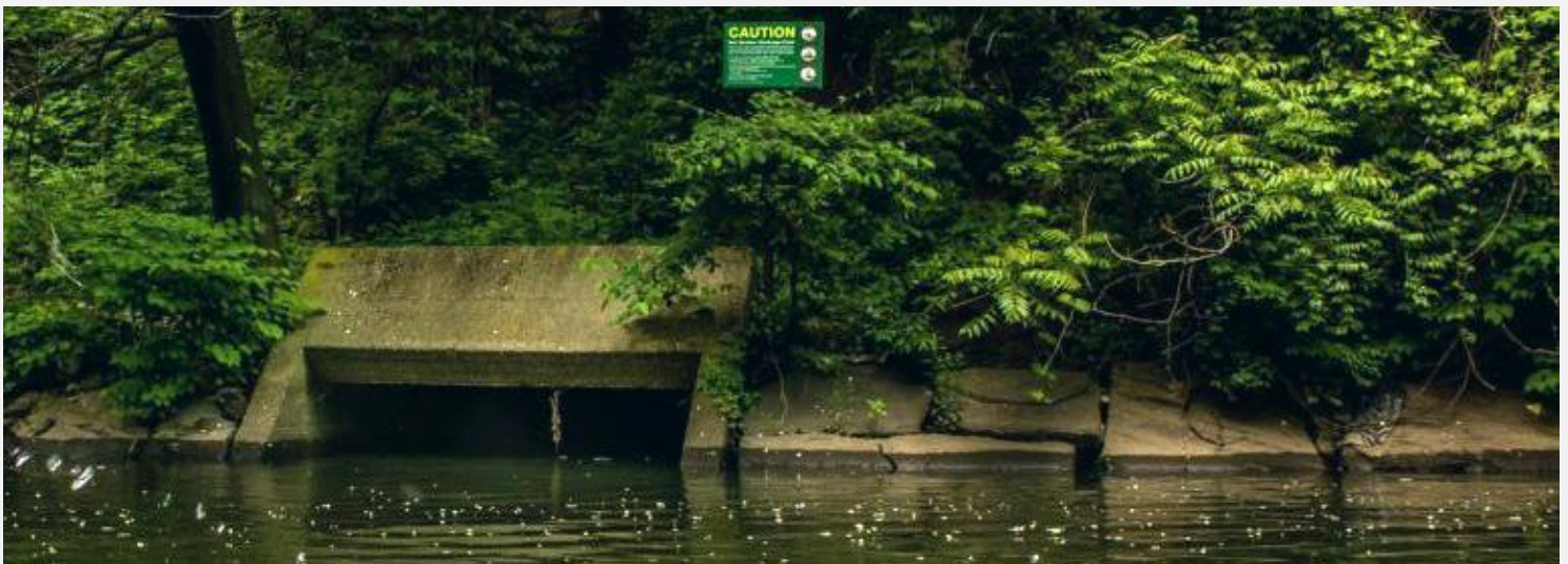
CSO discharge point on the Bronx River, Image: Adi Talwar
