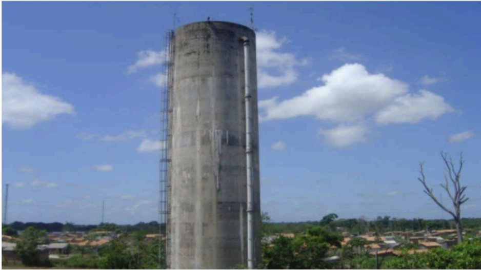
Appendix K – Photo of R02 illustrating the leaks (PMSB)
