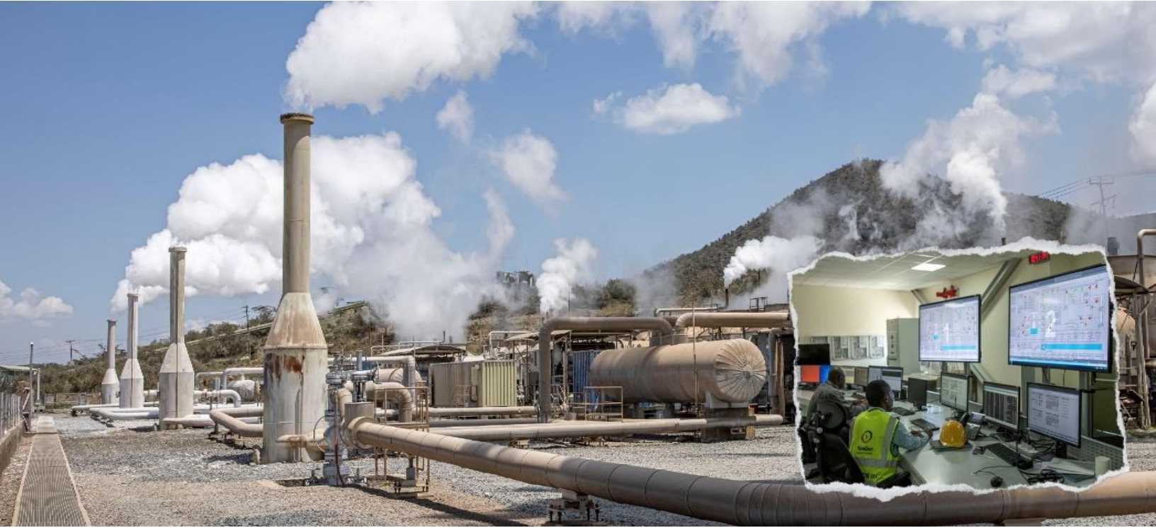
An image of geothermal infrastructure in Kenya.
